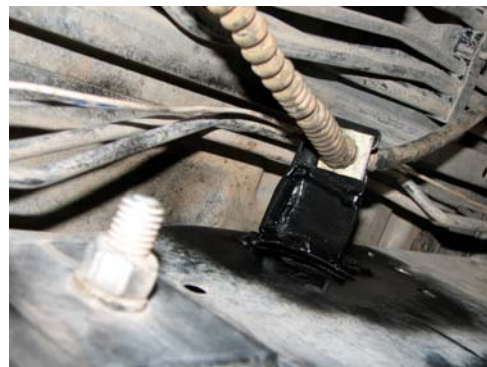
Front brake cable hanger, raised up.
